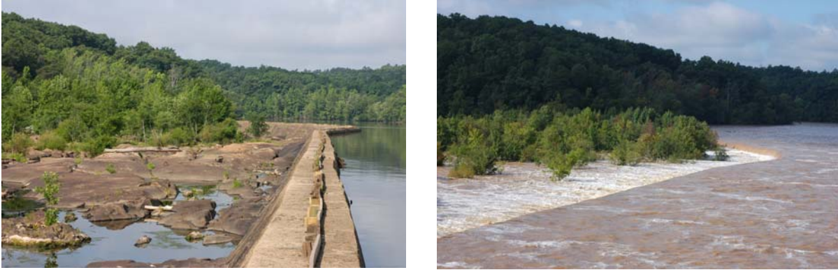
Figure 4. View of the Great Falls Diversion Dam under normal circumstances (left) and after torrential rains in the southern Appalachians (right).
