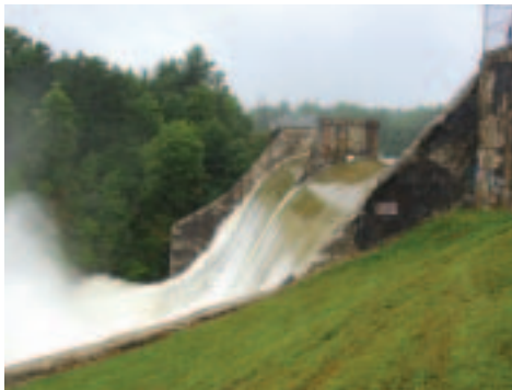
Catawba Dam Spillway – River flows were 150 to 200 times the normal amounts
