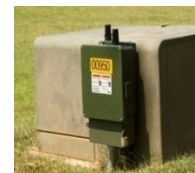
Underground Communications Box
