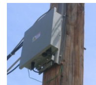
Overhead Communications Box
