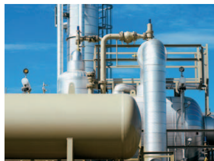
The Platteville facility is one of DEFS’ newest gathering and processing plants, built to process increased natural gas production in the Denver-Julesburg Basin area of Colorado.
