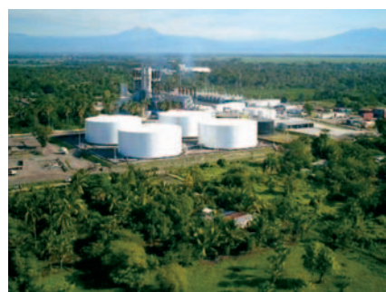
The 160-megawatt Planta Arizona in Guatemala generates electricity efficiently and at low cost, using dual-fuel technology.
